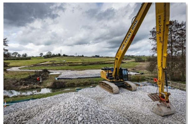
Figure 3: The T2G construction team lays the groundwork for a temporary bridge over the Great River Ouse, enabling us to efficiently move our internal construction traffic along our internal site access road.
