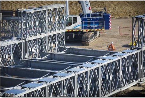
Figure 4: The image above shows our teams working to complete the installation of the temporary A422 bridge.
