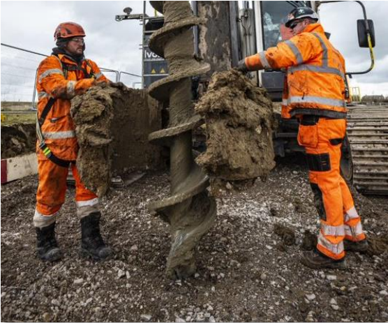
Figure 2: The T2G construction team working to ensure the safety and integrity of utilities, carrying out protection works to safeguard the local infrastructure.
