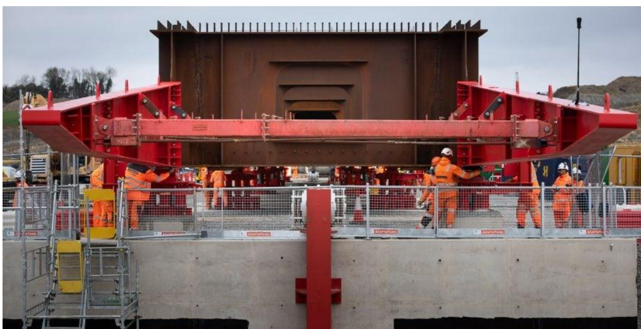
Figure 2: In the middle of March, the Westbury Viaduct team successfully pushed out the first 1,145 tonne beam into place, which now spans three piers. The beam was winched 135 metres at roughly 9m per hour and the process took around 11 hours to complete.
